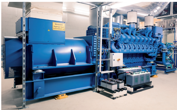
Diesel unit for emergency electrical supply if required
